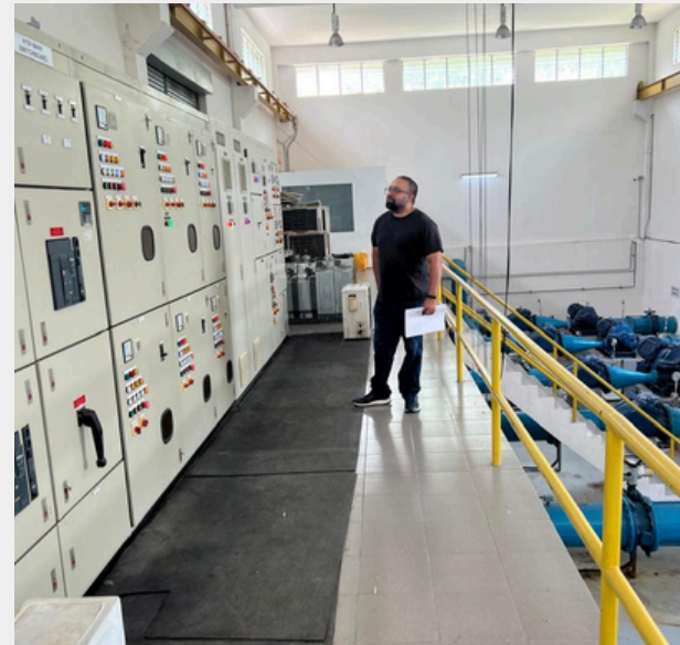
Pump House Monitoring 2023 - 2024)
